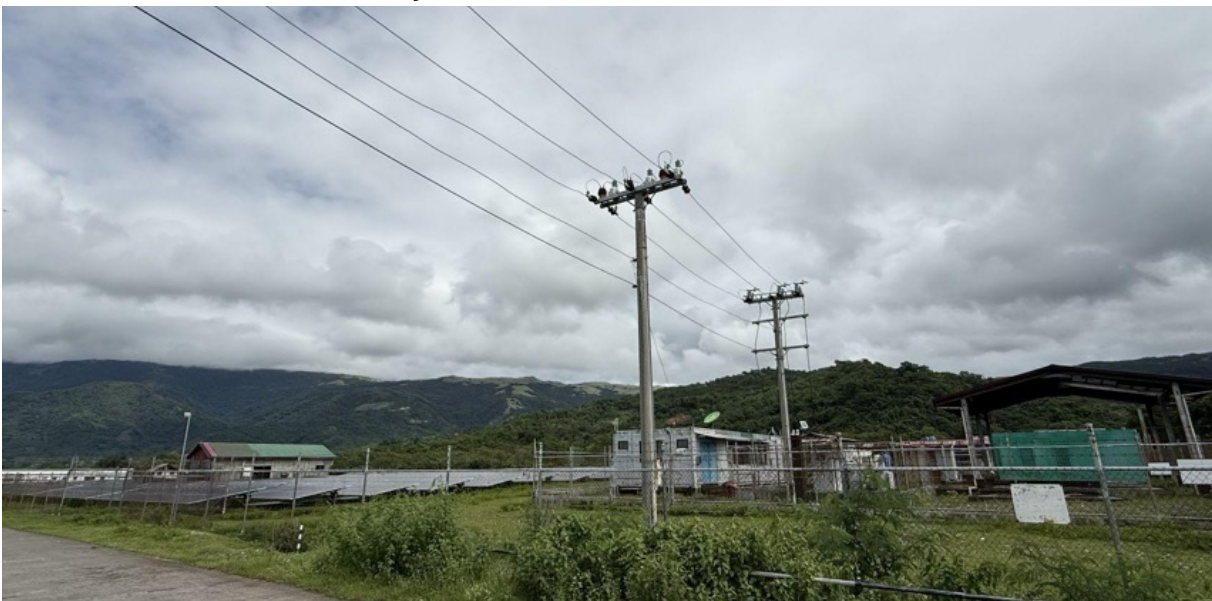
A 2MW backup diesel generator of the Solar Para sa Bayan project in Paluan, Occidental Mindoro. Source: CEED / Andoy Dimatulac
