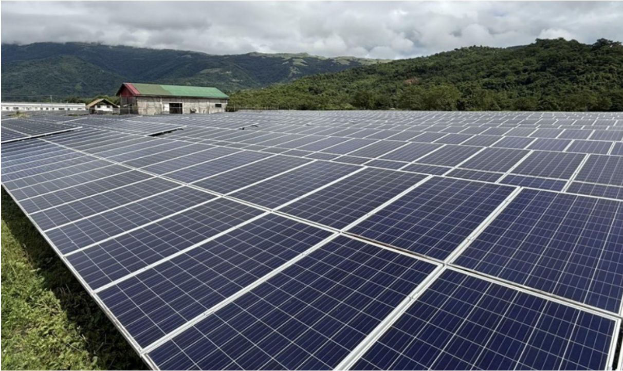
The abandoned 2MW solar farm under the Solar Para sa Bayan project in Paluan, Occidental Mindoro. Source: CEED / Andoy Dimatulac
