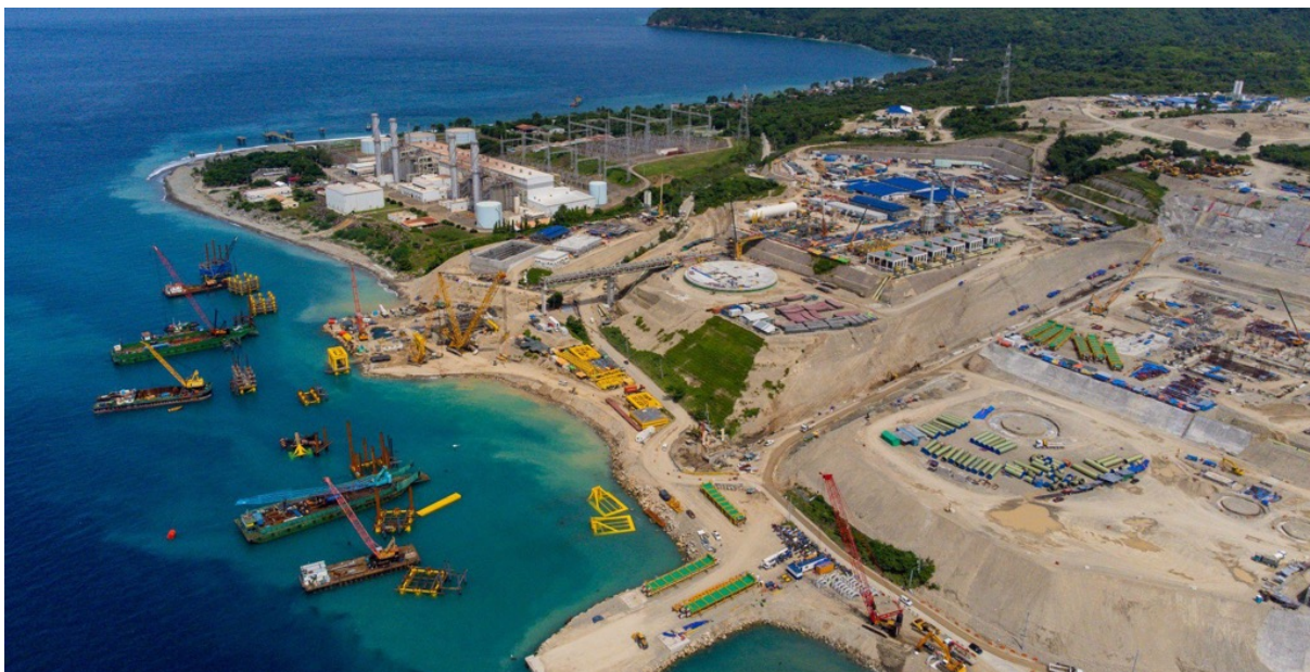
Photos of the project site taken through a drone last August 2022 show clearing operations have continued in spite of pending legal actions due to multiple irregularities. Construction activities are also visibly ongoing past the shoreline and into the VIP.
